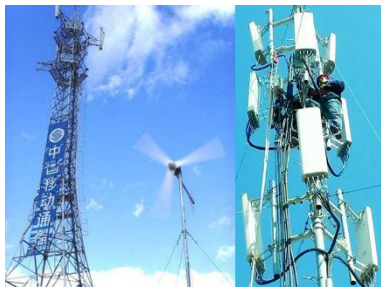
Figure 1: China Mobile builds the world's largest 8T8R 4G network
