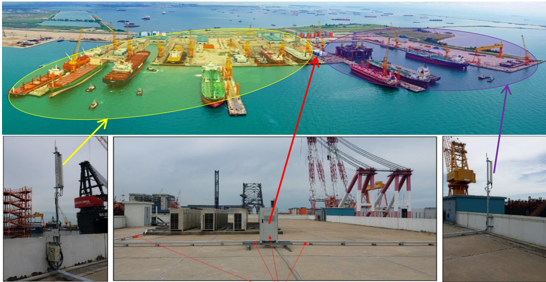
Huawei Cabinet, C-Channel, 150mmx 100mm and 50mmx50mm cable trunking as installed
