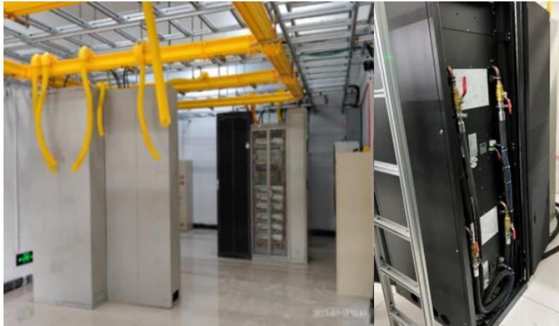
Figure 6.5. Application Case of Air-Liquid Mixing Cabinet for Energy Saving
