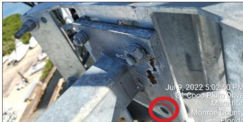
Example 2: Bolts missing from primary connection between mount standoff and collar connection to supporting structure.
